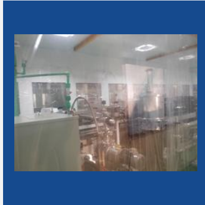
Walkable False Ceiling Services
