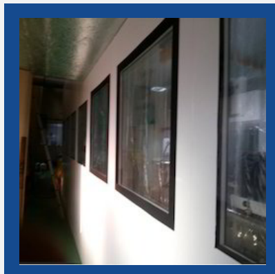
Modular Type Clean Room
